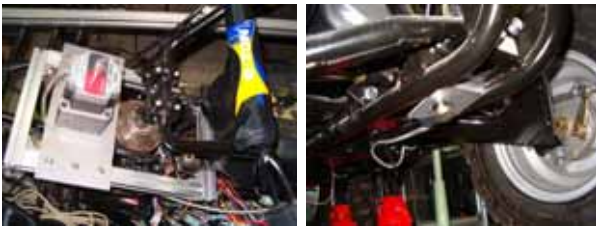
Photo. 2 Steering motor and position sensor
